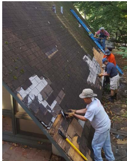
The Morales family removing layers of roof to A-Frame at Tower Hill.
